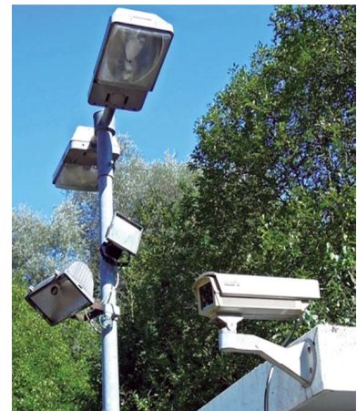
Fig. 3.9: Security lighting system with CCTV camera
